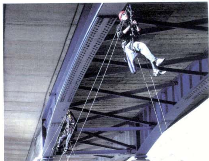
Roped access technicians carrying out steelwork inspection as well as the concrete bridge soffit
