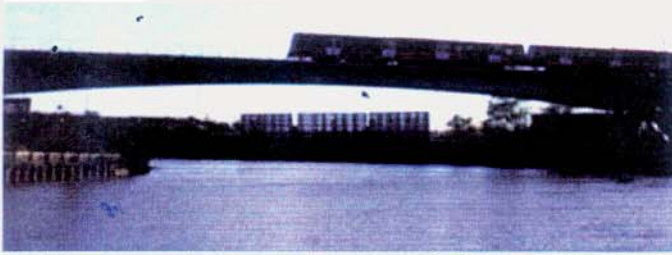
This large concrete bridge was the subject of a full conduction survey using roped access
